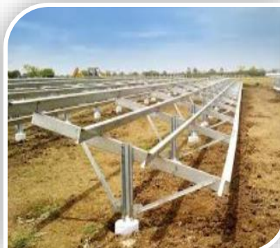
Solar Panel Structure
